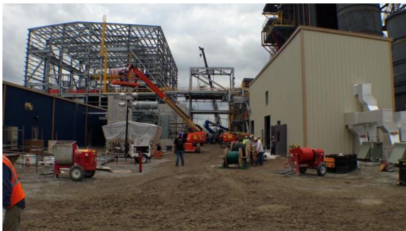
Construction continues on the Cane Run natural gas power plant construction site. Marty Pearl, Special to The Courier-Journal
